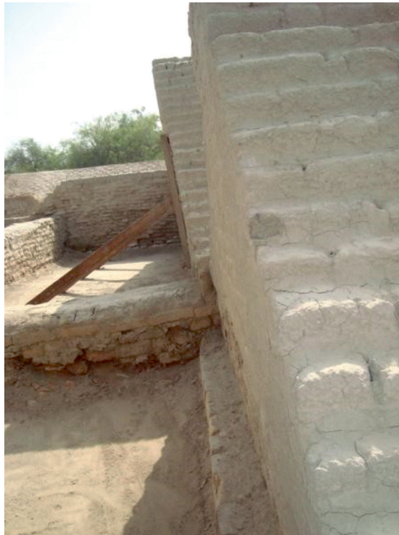
Figure 3: the view of the deformation
